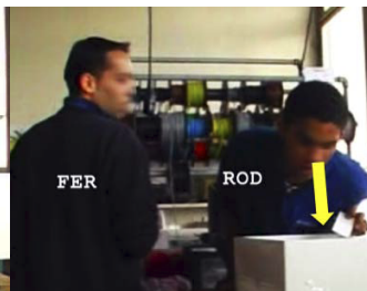
#2: ROD leans over the electric board and looks for the amperage of the main switch
