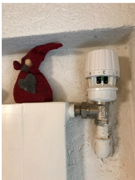
Picture 4. Valve to adjust the temperature of the radiator
