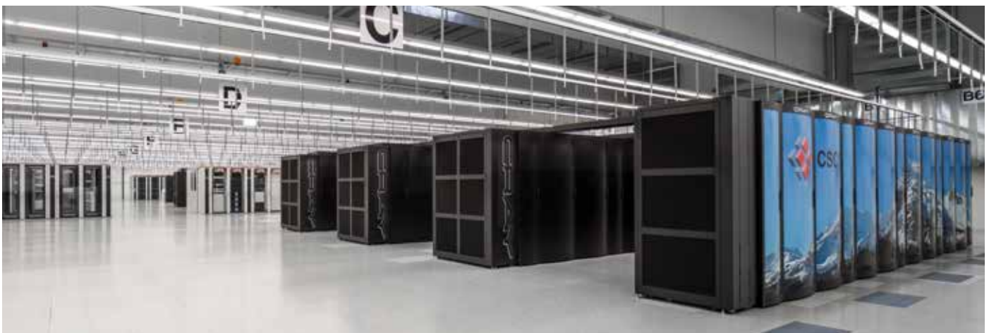
Figure 40 View of the machine room at the CSCS with cooling islands and the Piz Daint supercomputer on the right. Credit: CSCS
