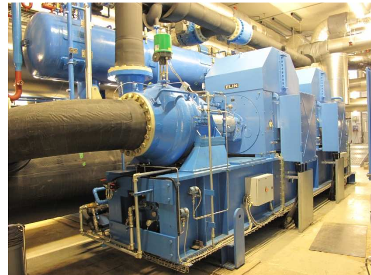
UNITOP 43/28 installed in the basement of SCANDIC hotel in Rolfsbukta
