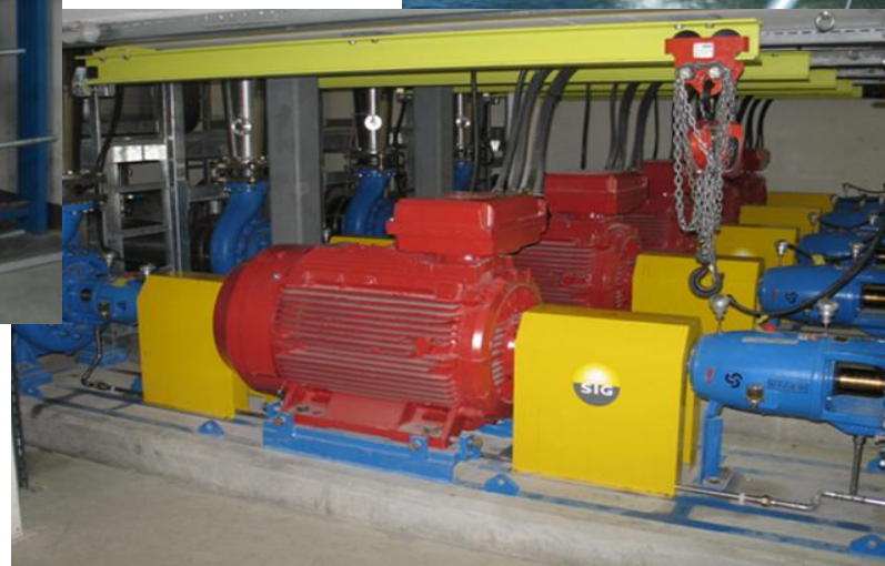
Station de pompage 4 x 700 m 3 /h + 1
